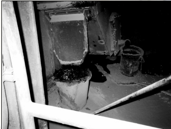
Mill Drainage – Pre Gear Shield
