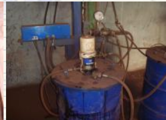
pump station maintained well
