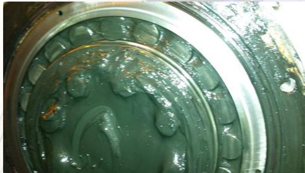
45 cm Inner Diameter Bearing from the Upper Pinion during inspection at 8,000 hours
